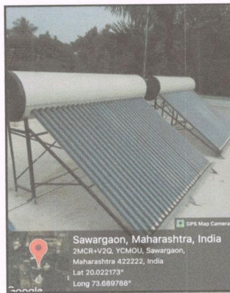
Photograph of Solar Thermal Water Heating System:
